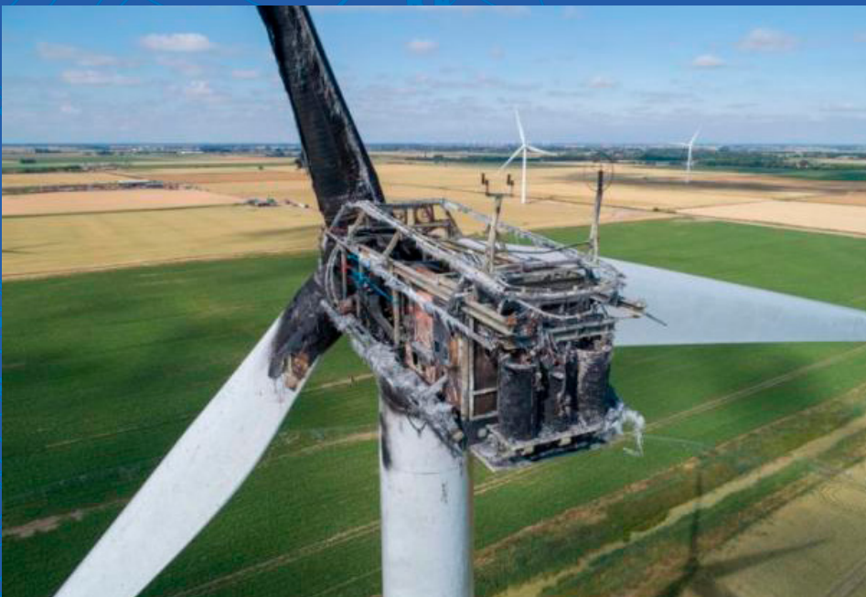
Damaged wind power plant
